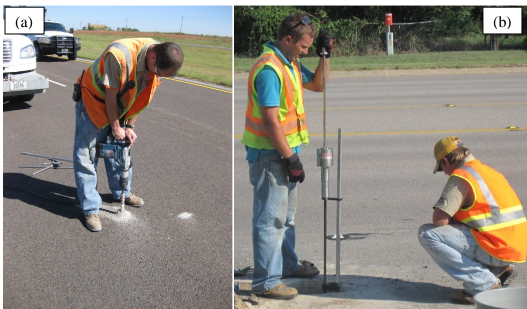
Figure 5. (a) Drilling a hole prior to DCP test, (b) dynamic cone penetrometer test
